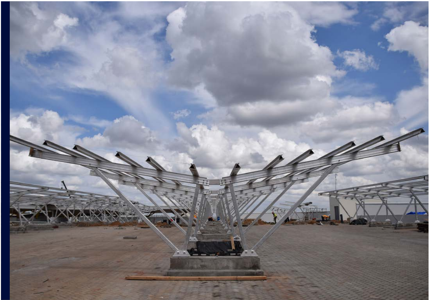
The Garden City solar project site in Nairobi, the largest solar carport in Africa and one of the largest commercial distributed generation sites in sub-Saharan Africa. Photo: CrossBoundary Energy
